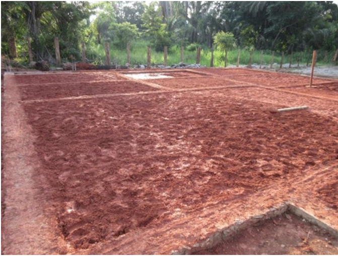
The foundations for the operating theatre, where the Parade funds will go in 2018
